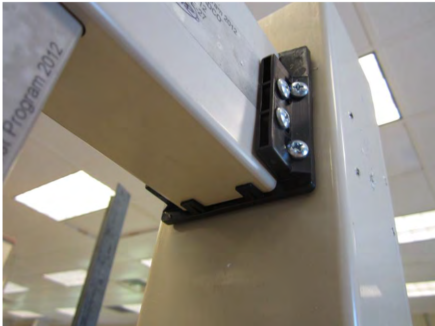
Photo No. 8 2 in by 3-1/2 in Top Rail-Bracket-Post Attachment
